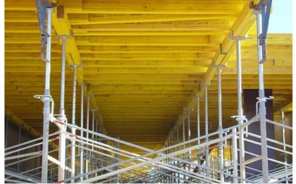
LVL Beams used in conjunction with Sta-Flex on The Villa
